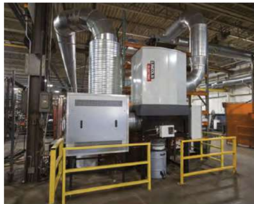
Push/Pull System installed at Elgin Sweeper Company
